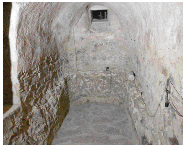
99. The lower ground of a U-shaped tower of the late Roman fortress is preserved completely in a cellar of an old house in the town of Mautern (Austria)
