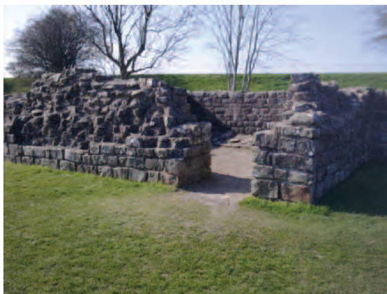
130. Turret 52a (Banks East) was one of the earliest parts of Hadrian's Wall to be taken into state care in 1933
